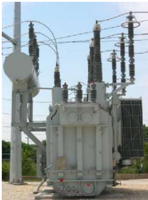
Fig: Power Transformer
