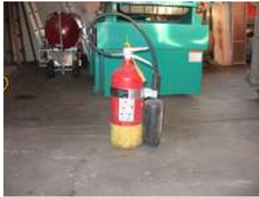
Carbon dioxide extinguisher
